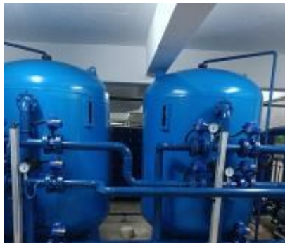
Rainwater Recycling System in Vietnam
